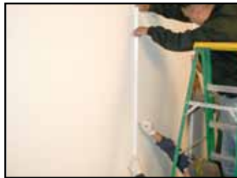
2 Layout and mark holes for the first End Snap Bar, making sure it is plumb. All further dimensions rely on the first bar.
